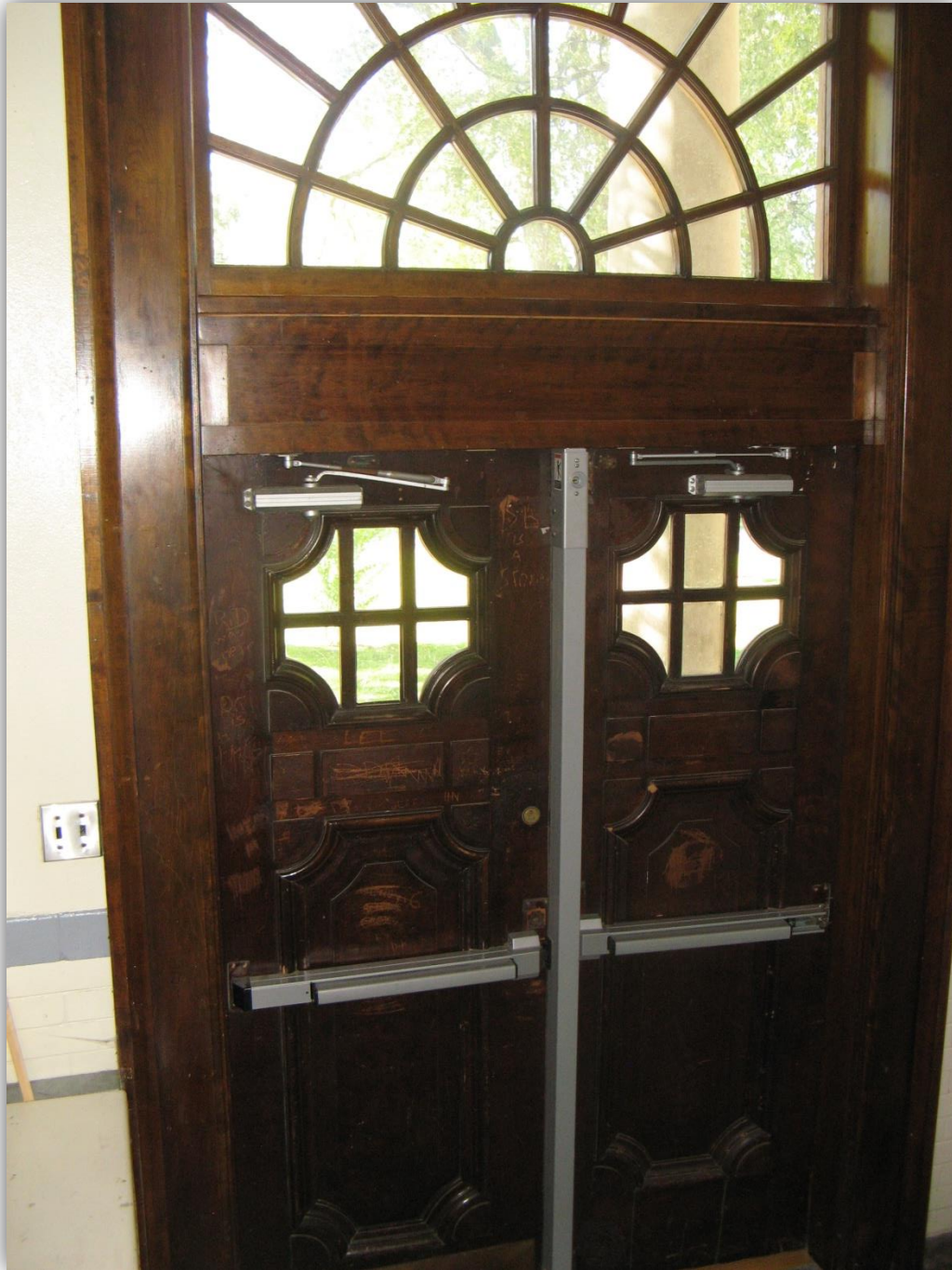
Date of Photo: Oct 2016 View: Interior door front entrance. File Name: RCBHS 2016-5 Credit: K. Ratcliffe
