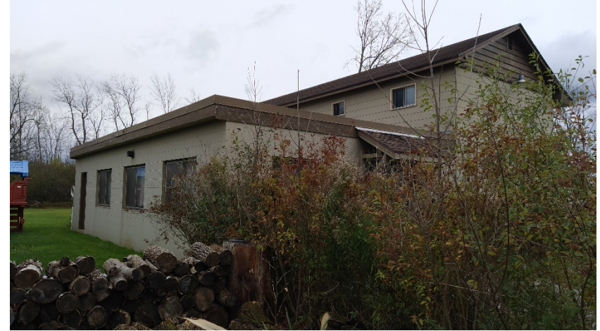
View of a portion of the northwest elevation of Site Building 2 on the Subject Property, looking southeast.
