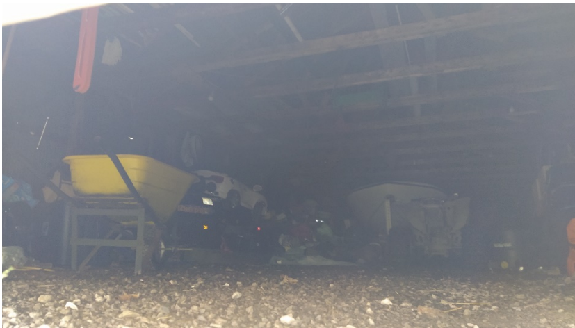
View of the interior portion of the storage structure of the Subject Property.
