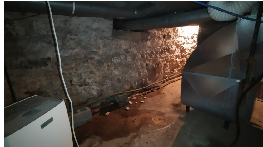
View of the natural gas fired furnace in the basement of Site Building 1 of the Subject Property.
