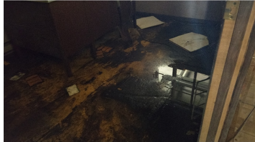
View of the apparent water infiltration within the first floor garage area of Site Building 2.
